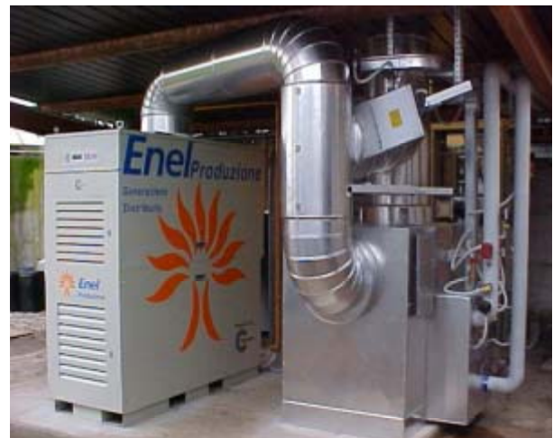
Figure 8. – C60 CHP System at Bauli Restaurant
