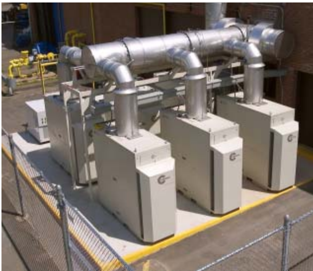
Figure 12. –UTC Power’s PureComfort 240M
