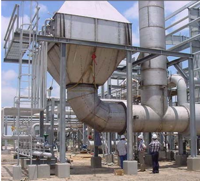
Flue Gas Heat Exchanger (EX101)
